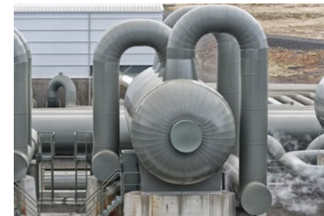
• the water supply pump station
