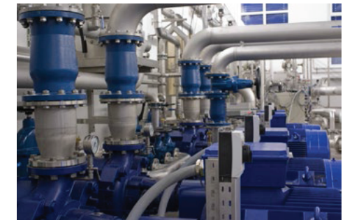
• The city concentrated water supply
